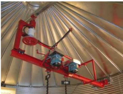
A stirring machine used for in-bin drying
