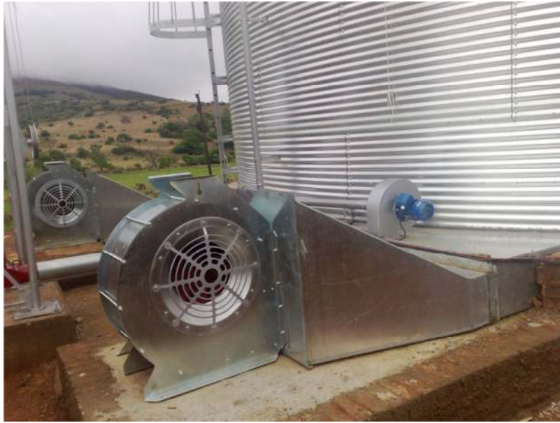
Aeration fans with small fumigation fan.
